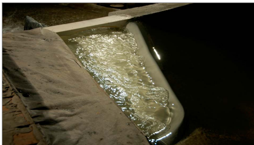
Fig. 11. Spillway work under conditions of the discharge passage of about 400 \text{m}^3/\text{s} (change III)
