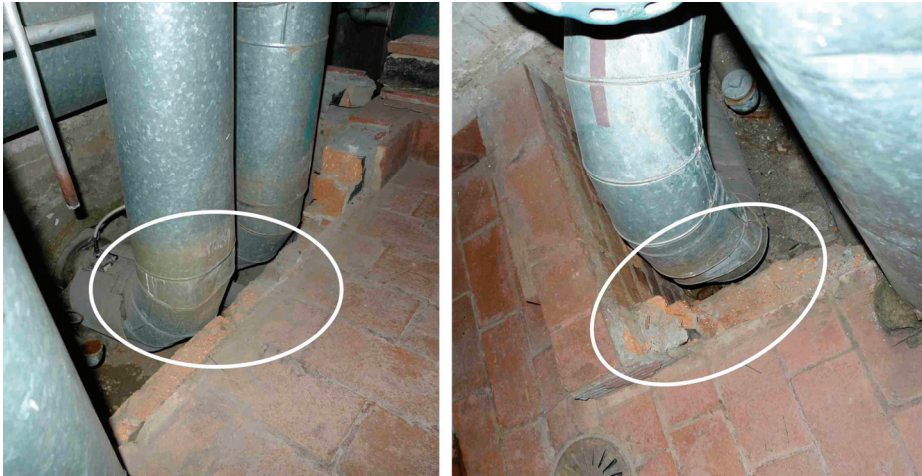
Fig. 16. NH boiler room. Visibly bent pipes and incuts made to protect the piping from damage
