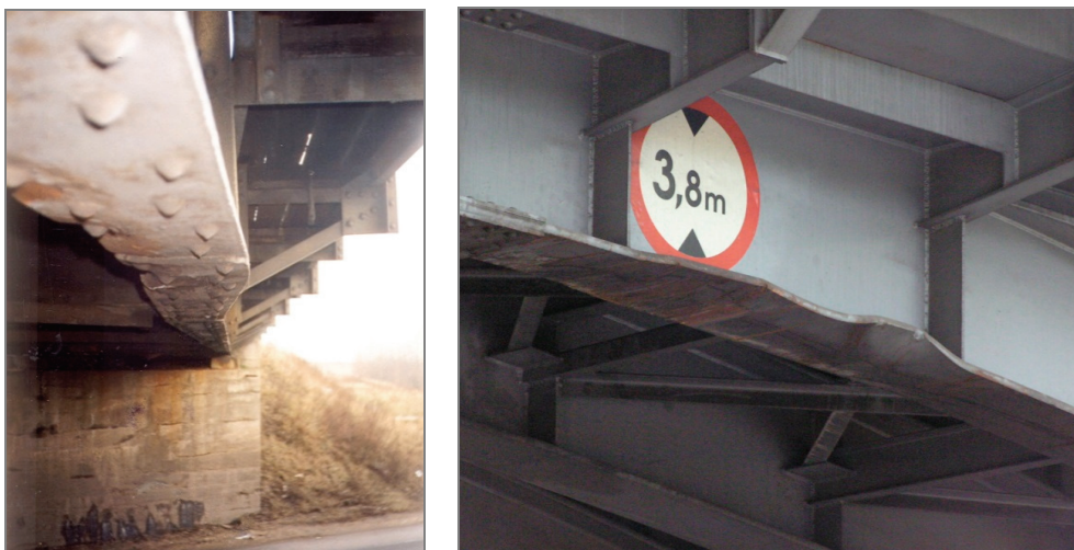
Fig. 2. Deformations of bridge plate girders
