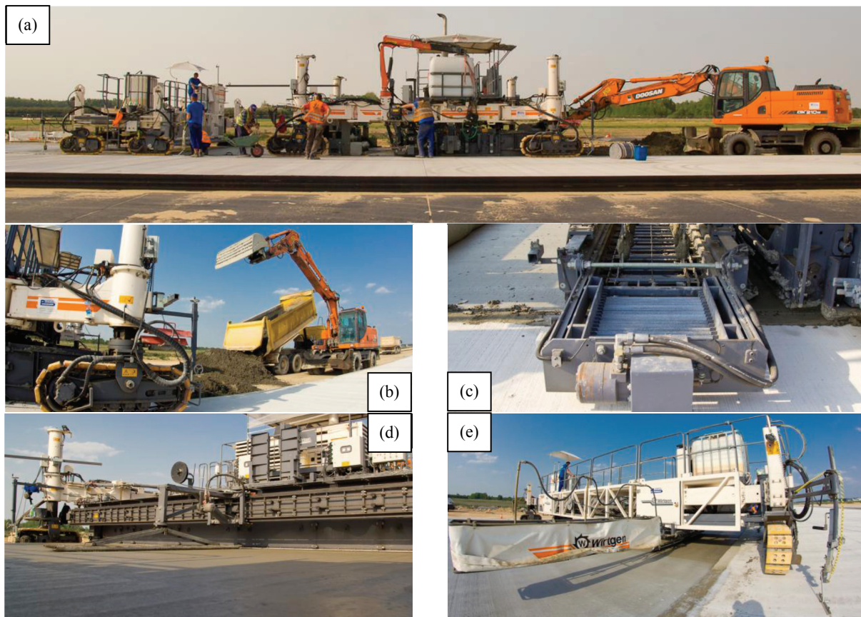
Fig. 6. Construction of a concrete abrasive layer of runway in Pyrzowice, (a) view of 3 parts of band laying machine and excavator, and consecutive concrete laying phases: (b) concrete mix supplied for preliminary spreading with the excavator, (c) element of second part of the spreader placing dowels at the width of the band made, (d) waterproof layer sprinkling system, – view of laying the second band of abrasive surface [own study, on the basis of [17]]
