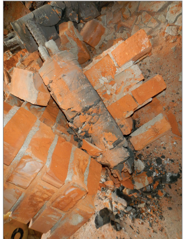
Photo 14. Damaged masonry foundation specimen
