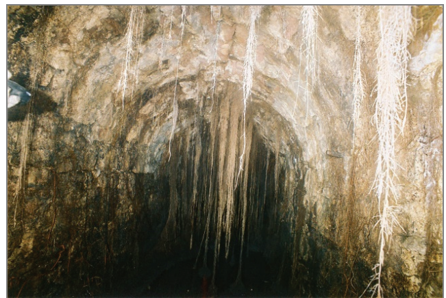
Fig. 3. A view inside the adit with roots overgrowing the support wall (Photo: W. Preidl [14])
