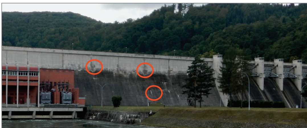
Fig. 2. View of the inspected downstream wall of water dam in Rożnów with circled example fragments affected by surface change
