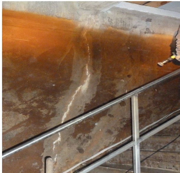
Figure 6: The exemplifying crack with salting out in the longitudinal partition wall.
