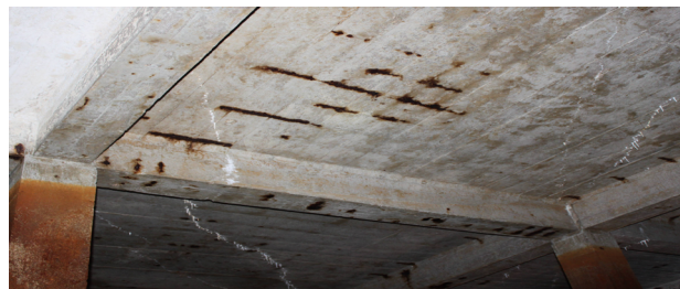
Figure 7: The exemplifying crack with stalactites of salting out in the roof slab.
