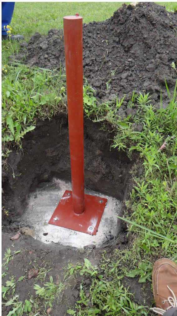
Figure 12: The structure of controlled point whilst fixing to the upper surface of the roof slab.
