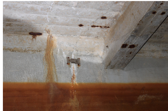
Figure 10: The crack width gauge fixed to the longitudinal partition wall.
