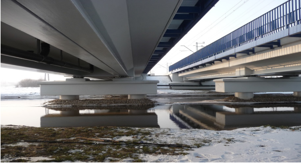
Figure 36: Bottom view of “Wiarna Rzeka” bridge.
