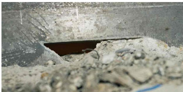
Figure 19: Plastic deformations of steel dowels in the region of the sharp notch in the SA shape (push-out specimen [30]).
