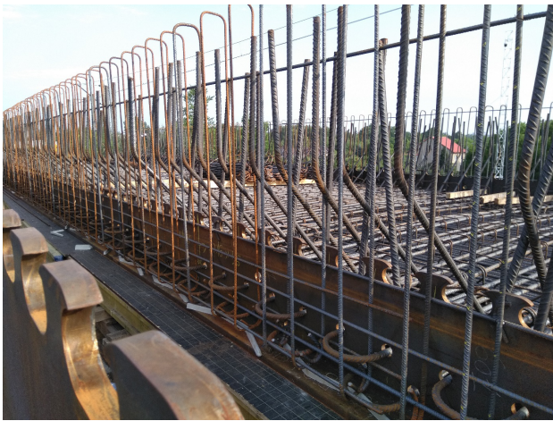
Figure 14: T-sections and reinforcement of bottom part of the superstructure (main stirrups crossing concrete dowels are still missing at this stage, compare Fig. 9).
