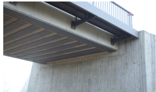
Figure 2: The idea of external reinforcement by SSF Ingenieure applied in the trough girders (both in the longitudinal and transversal directions of the slab for railway bridges) in the bridge located next to Spergau [9, 1] (picture by Guenter Seidl).
