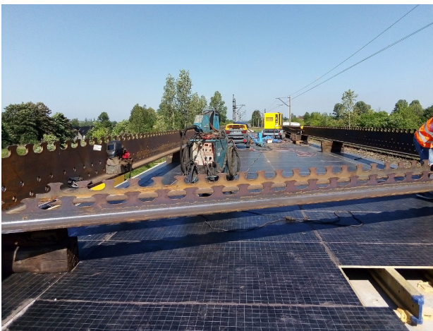
Figure 12: Steel structure after welding (picture by Nowak Mosty): main elements and transversal elements at the edge of slab.
