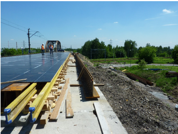
Figure 11: Steel T-sections on site next to scaffolding prepared for in situ slab (picture by Nowak Mosty).
