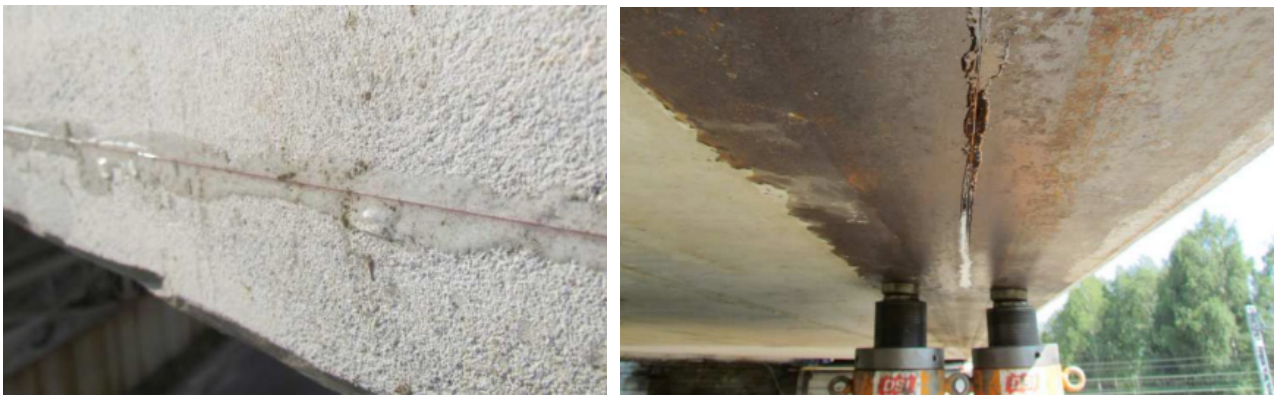
Figure 21: Optical fibers (light wires) on concrete and steel.
