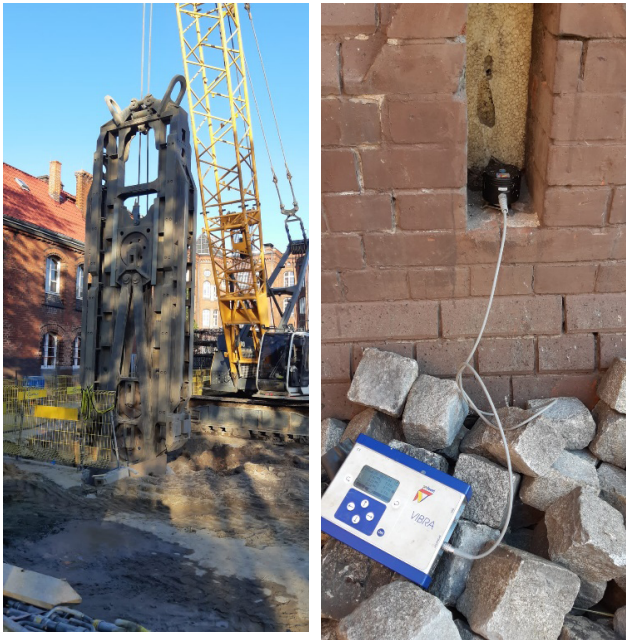
Figure 4: The examined case: structure sensitive to dynamic excitation located in the vicinity of diaphragm wall installation (a); vibration monitoring made on structure (b).
